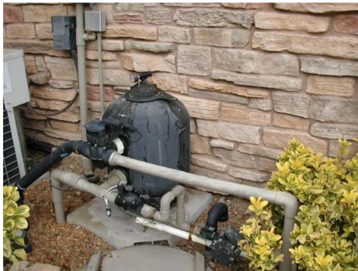
Figure 2-2. Graywater Reuse System (ReWater®) in Escondido, CA (existing system).
